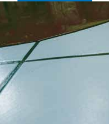
Detail of the application of Ultraplan on an existing ceramic tile floor after the application of Eco Prim T Plus
