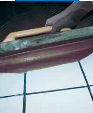
Application of Ultraplan with a metal trowel on an existing ceramic tile floor after the application of Eco Prim T Plus
