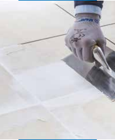
Levelling off and sealing the joints in existing ceramic floor tiles with Planiprep 4 LVT
