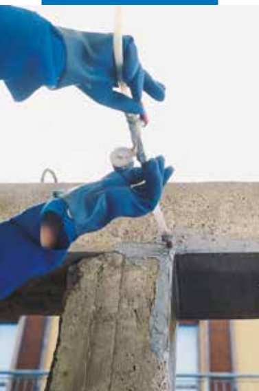
Column clad with Adesilex PG1
