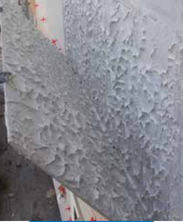
Excellent wetting between the substrate and the back of the tile
